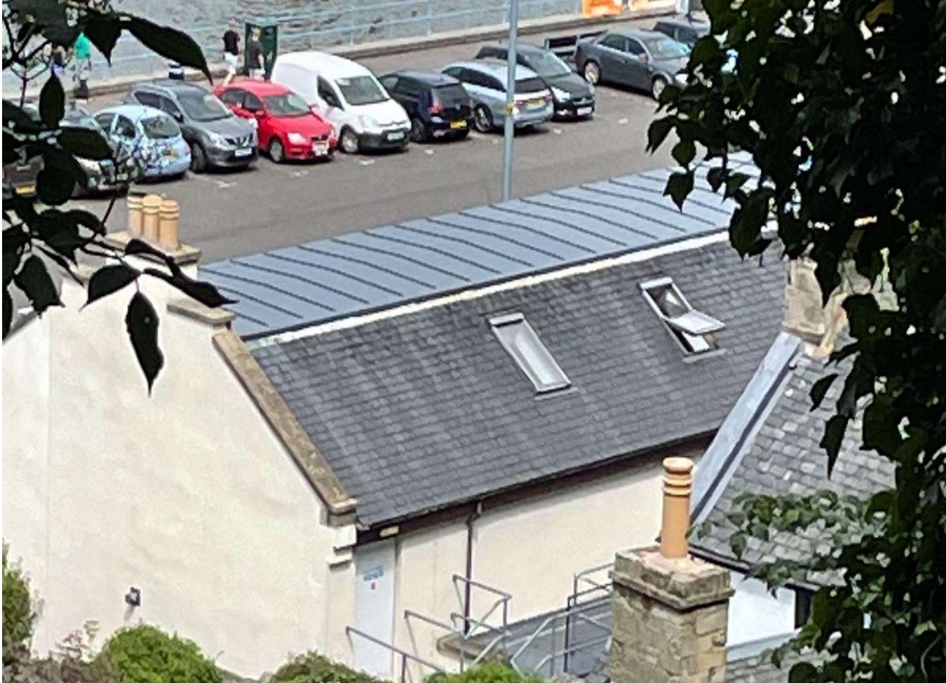
(c) 4 Newhalls Road - Unknown when the work in this photo was done
